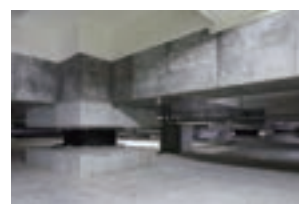
Seismic isolation equipment of the Disaster-Resistant and Eco-Friendly Warehouse (Ibaraki Distribution Center No. 4 in Osaka)
